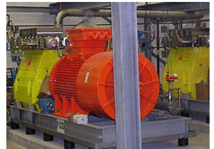
Process pumps to pump salt water extracted from crude oil back to source
